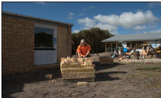
Above: Luke Green, local Aboriginal community member working on the three constructions in Munro Place, Whitemark.
