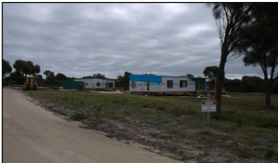
Above: Two new homes currently under construction on Thunder and Lightning Bay Road.
